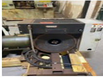
#727 • Sullair ES-8 Rotary Screw Air Compressor Missing Motor
