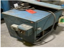
#582 • Unmarked Air Filtration System Unmarked Air Filtration System
